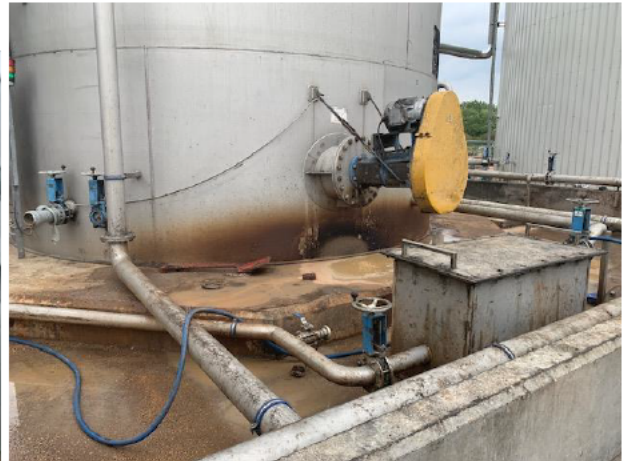
Image 2 – Leaking effluent tank
