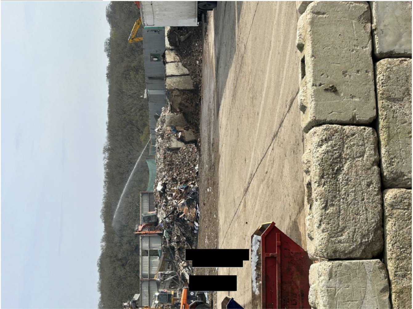
Photograph 1 illustrating pile lengths and widths which are exceeding Table 4.1 and, in the layout and fire plan drawing No THEO-3483-03.
