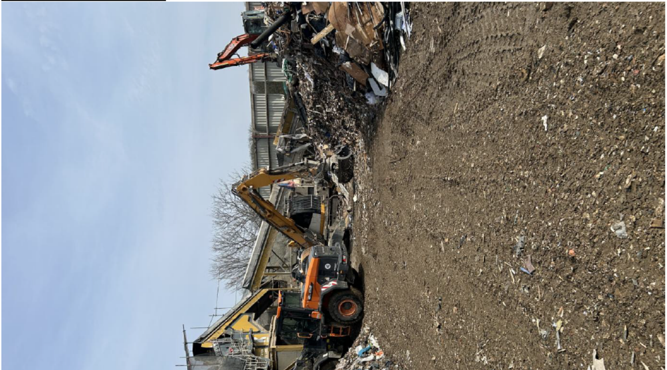
Photograph 2 illustrating pile lengths and widths which are exceeding Table 4.1 and, in the layout and fire plan drawing No THEO-3483-03.
