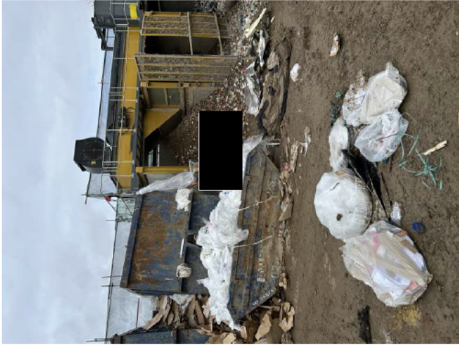
Photograph 7 illustrating waste being stored/processed outside permitted boundary
